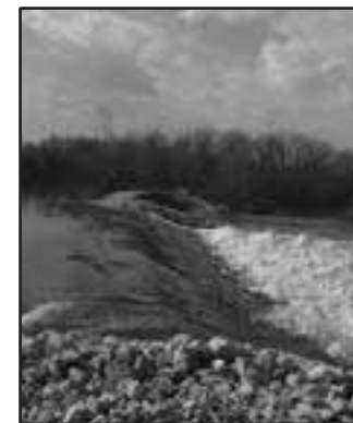
Flood water pouring over the newly constructed Barkhausen Levee in November of 2009.
